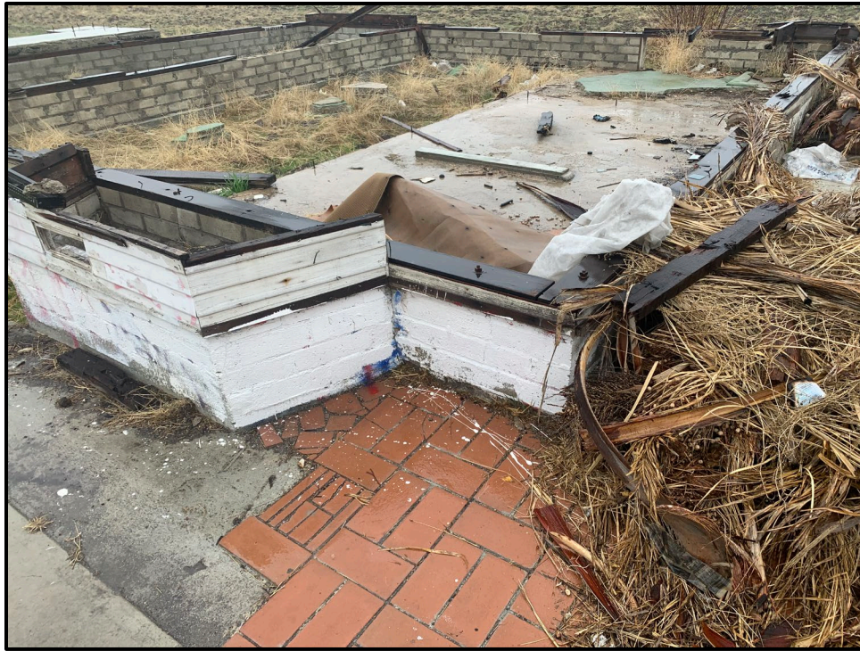
Plate 3.2–18: Overview of the foundation for the single-family residence, showing the bay window, facing northwest.
